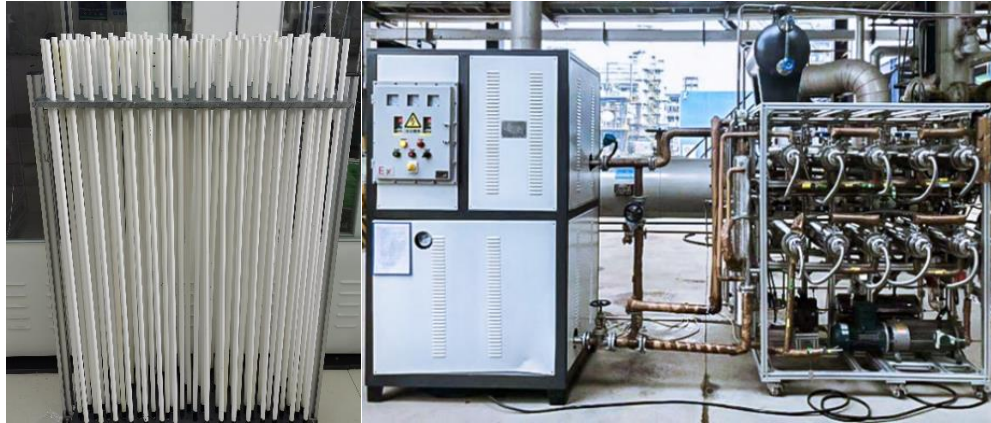
Photos of one-meter-long tubular MFI zeolite membranes (left) and pilot-test membrane system (right) for on-site butane isomer separation at Shandong Chambroad Petrochemical Co., Ltd in Boxing, China.
